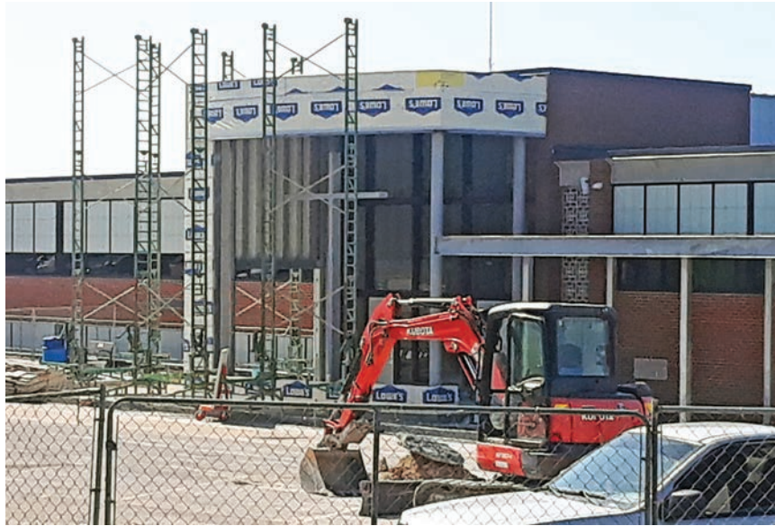
Work progresses on the upgraded "Crucifix Entrance" to Helias Catholic High School, 1305 Swifts Highway in Jefferson City, on Aug. 3. Completion of the project and upgrades to the school's James Rackers Fieldhouse is scheduled for late fall.
