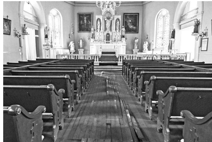
Floorboards damaged by floodwater at the Old St. Ferdinand Shrine in Florissant, Mo., are seen July 26.
